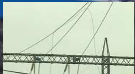
The cause of all the trouble, a small earth wire that broke in the wind and crossed the cables going into Auckland city
